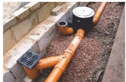
Underground Drainage System
